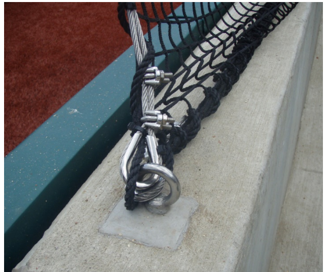
Figure 5. Bottom Cable Termination
